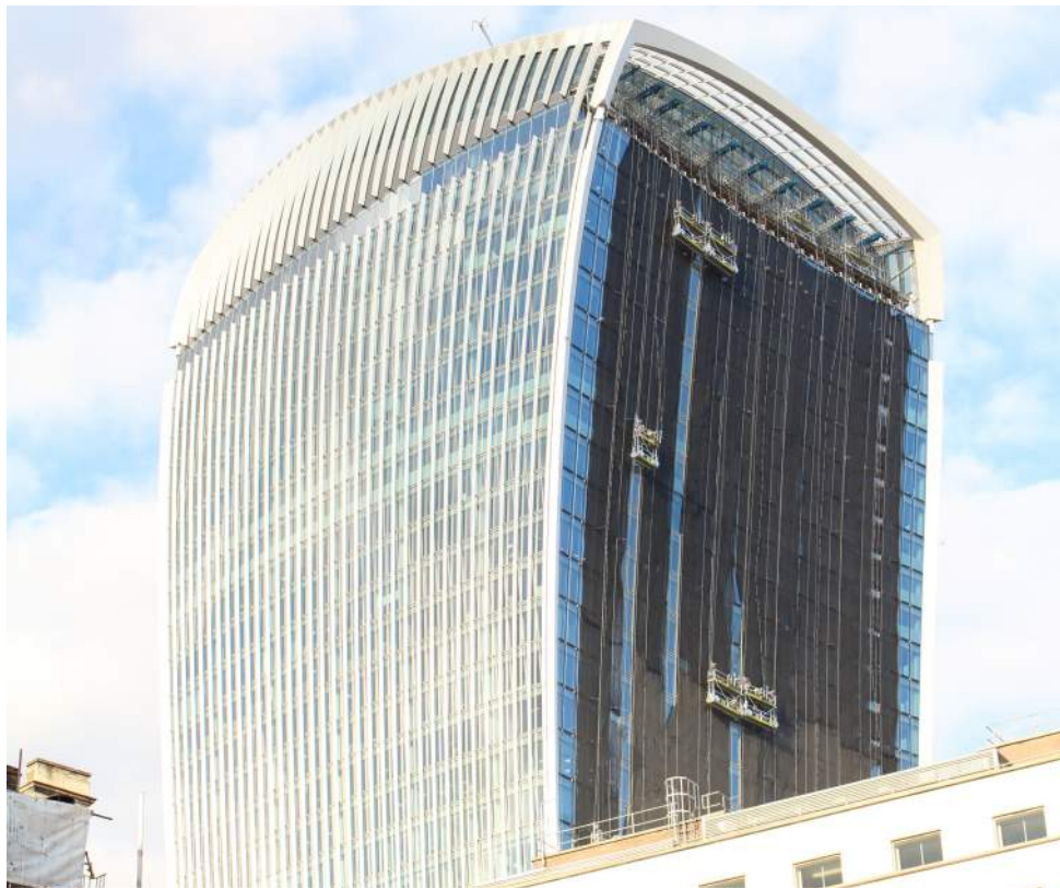
Figure 9: Photograph of a brise-soleil being installed on the “Walkie Talkie” building (20 Fenchurch) in London, UK. (Photo courtesy of Albert Brooks.)
