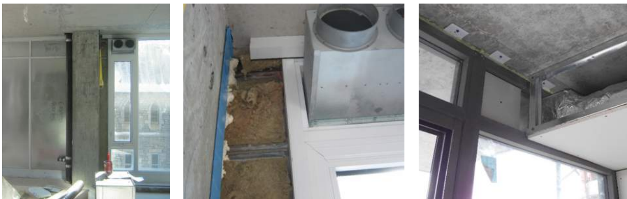
Figure 4: Examples of interference/lack of coordination between structure, mechanical services and window wall systems.
