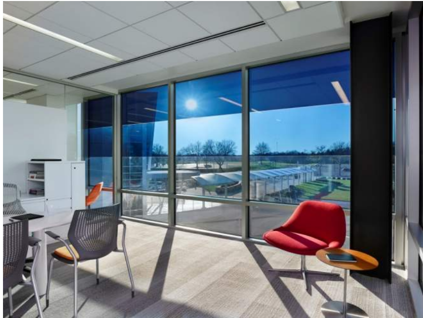
Figure 4: An example of zoning of electrochromic glass in a vertical glazing application. In this case there are 4 zones – top row, middle top row, middle bottom row and bottom row. There are actually only 2 separate EC panes, since the top EC pane is separated into 3 independently controllable zones (in-pane zoning). In this instance the top zone is fully tinted to 1%T to control the glare, the bottom zone is in the highest transmission state (60%T) to control light color quality, and the middle zones are at appropriate transmissions (6%T and 20%T) to manage heat gain and tune the daylight admission. Photo © Jeffrey Totaro, 2015.
