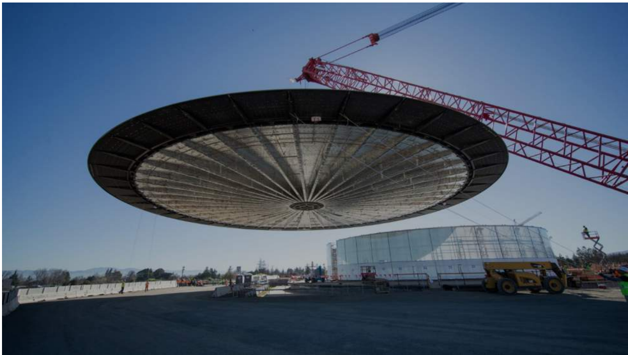
Figure 32.: This composite steel and carbon fiber roof is being fitted on all glass walls at the new Apple Headquarters in Cupertino, CA. The composite roof is fitted to the glass with very little room for error. The entire construction is fitted onto the roof of a reinforced concrete building. (photo courtesy of Apple/Digital Trends)
