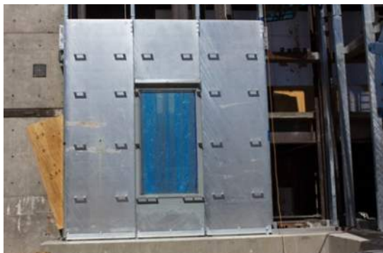
Figure 3a: Installation of SSCW test structure: First floor cassette showing FE/BR window and ballistic steel plate prior to installation of granite cladding
