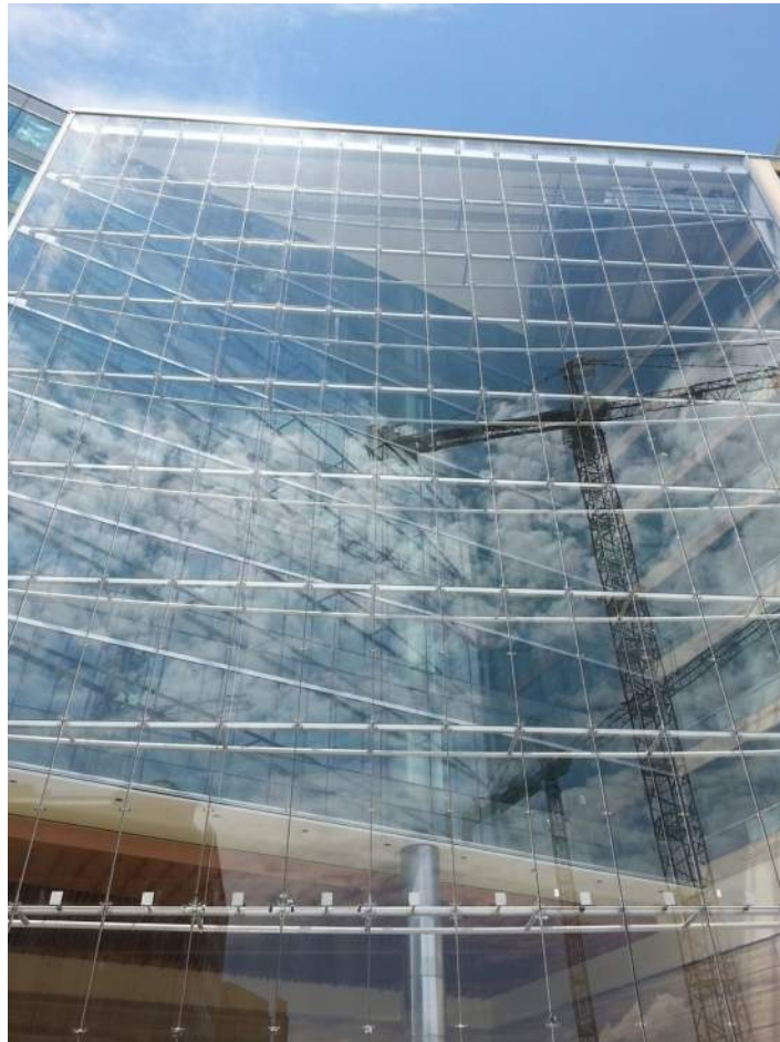
Figure 30. 31M long steel trusses provide the wind load support for the lobby at 601 Massachusetts Avenue in Washington DC. The steel trusses were machined after fabrication to insure the dimensional accuracy of the glass attachment points and the pin to pin length of the truss itself. (photo courtesy of W&W Glass)
