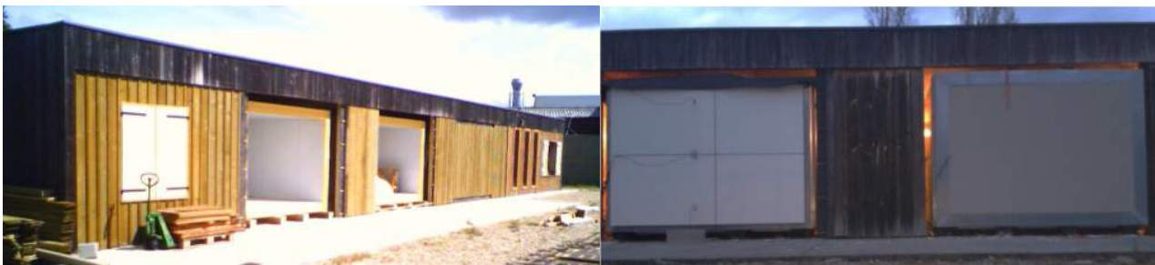
FCBA Experimental platform, empty cells and mounted walls (Trespa® ventilated façade & EIFS)
