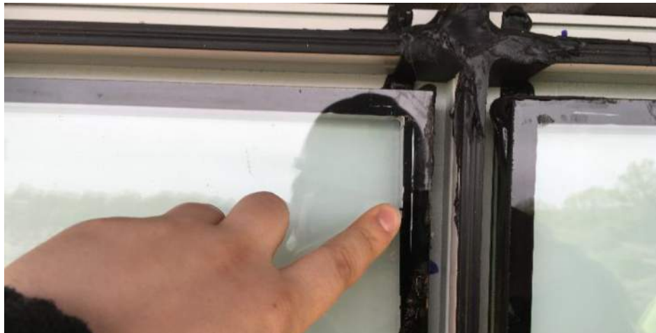
Figure 1: View of a skip or discontinuity between the primary and secondary seal of the IGU
