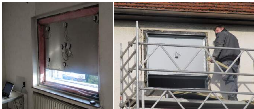
Figure 6: The shadow box mockup with sensors from the interior (left) and from exterior without glass (right)
