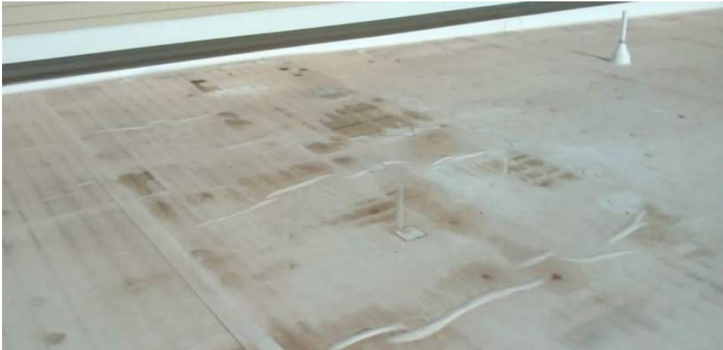
Figure 4: View of a poorly installed waterproofing membrane.
