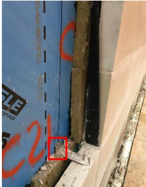
Figure 2: View of a poorly attached insulation in a wall cavity with missing seals at anchors.
