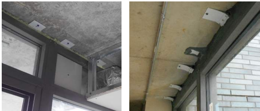
Figure 3: Examples of strap anchors at the head rail of a window wall. Left, straps secured with concrete screws to the underside of the floor slab with one component polyurethane foam air sealant foam in the rough opening gap as an air seal. Right, rough opening gap exceeds the length of the strap so straps are extended by stitching end-to-end. A gunned sealant was applied over the foam to ensure continuity of the air barrier. Encapsulating the perimeter of the straps may be needed if access behind the strap for sealant application is restricted.
