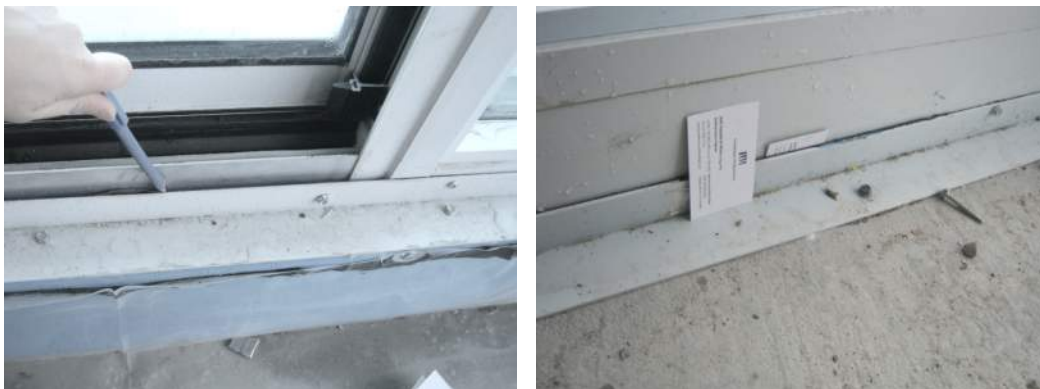
Figure 6: Careful thought in 3D is required to ensure continuing of air and water leakage control.
