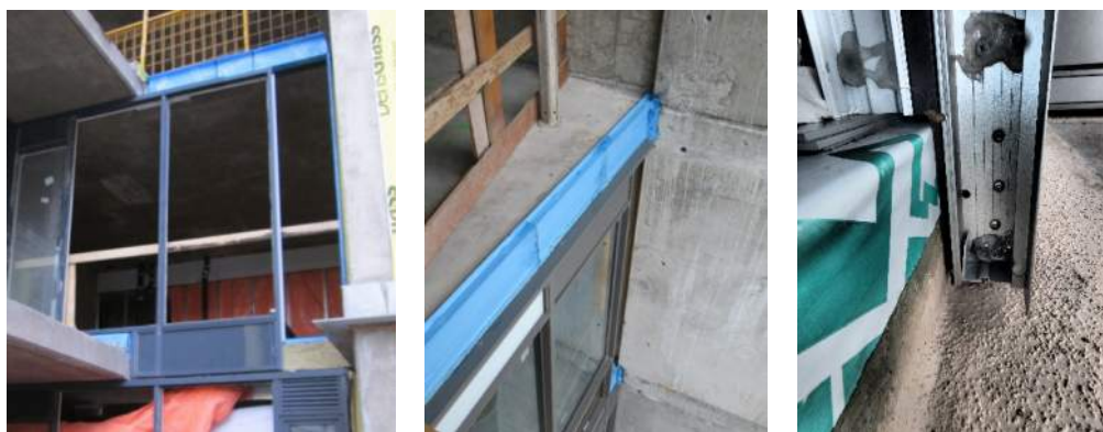
Figure 2: Canadian window wall system during installation. Left, story high panels have been installed with the other half of the frame extended to cover the floor slab.
