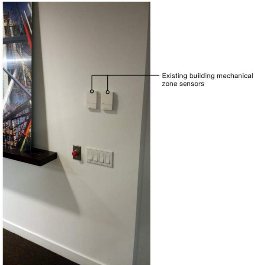
Figure 3: Existing building sensor placement - clustering
