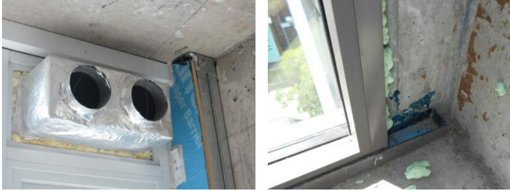
Figure 7: Careful thought in 3D is required to ensure continuing of air and water leakage control.
