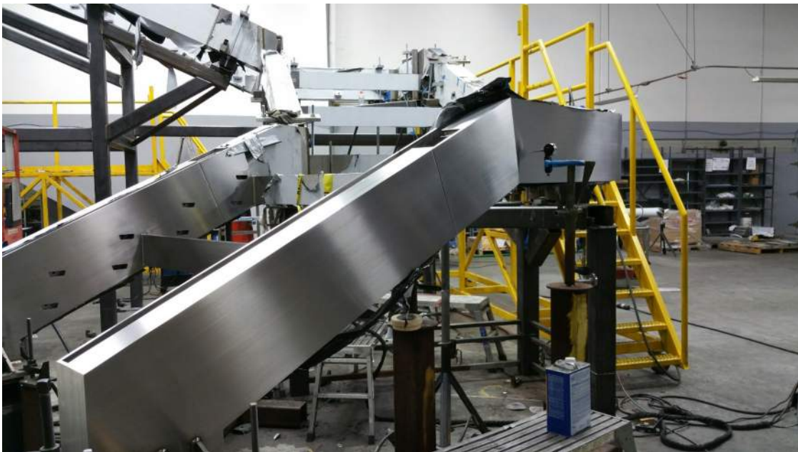
Figure 11: The stringer assemblies for a glass and SS stair for an office space in Beverly Hills. Note the dial indicator to monitor deflections as the unit is welded together. (photo by the author)
