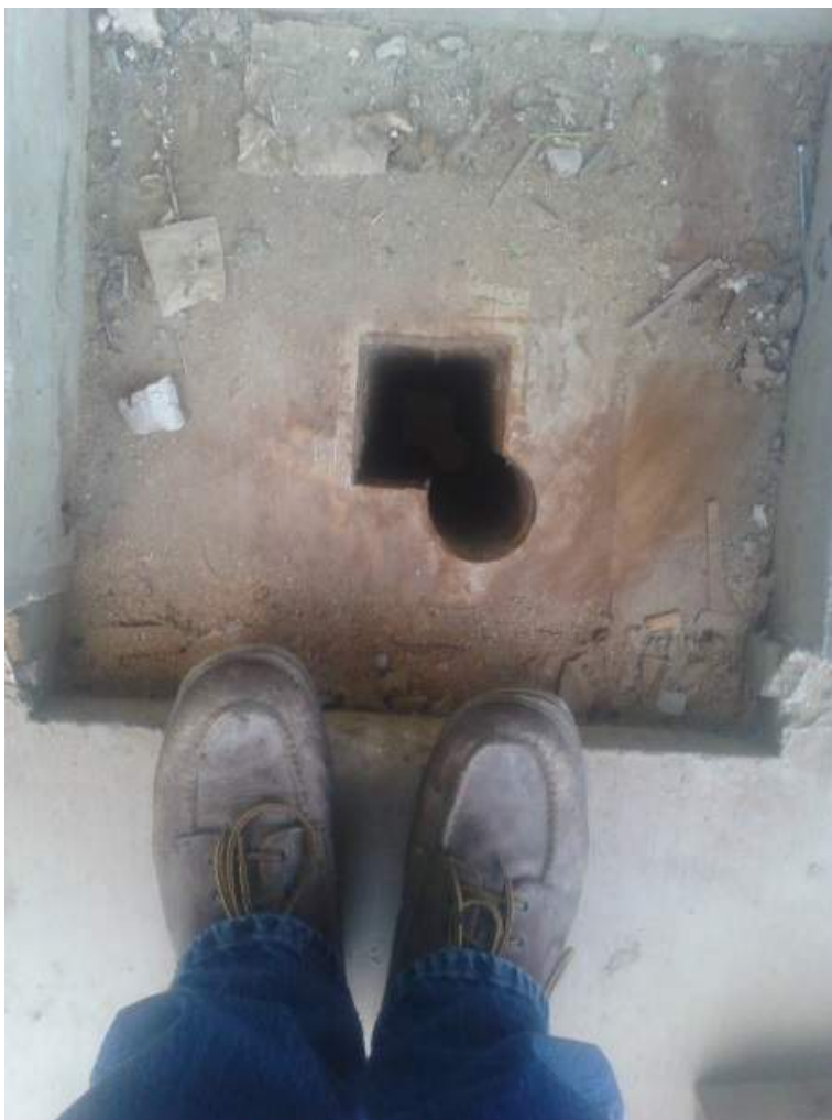
Figure 27: This 4x4TS was meant to be cast in the location that was later core drilled. (photo courtesy of W&W Glass, LLC.)
